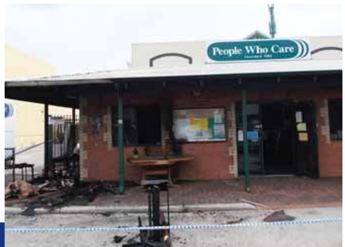
The fire damaged front of the PWC Guildford Office
